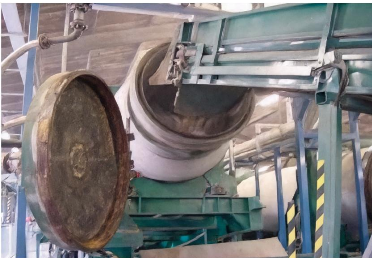
FIGURE 5: Autoclave for thermal treatment of MSW to RDF.
